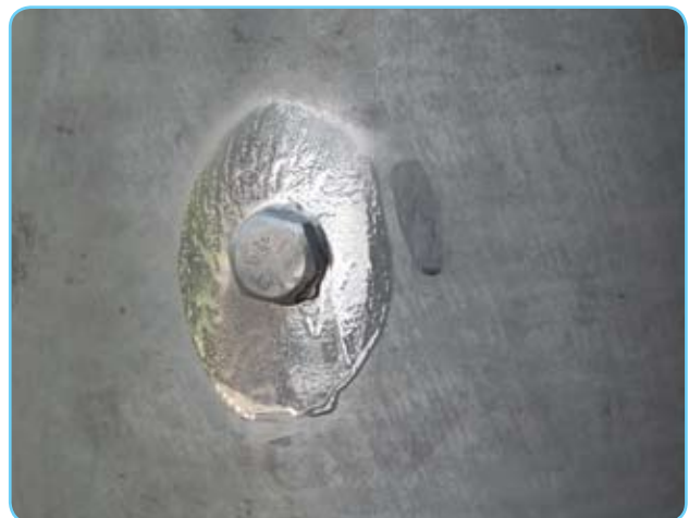
Zinc rich paint used on the new hole and plastic plug fitted to seal the hole.
